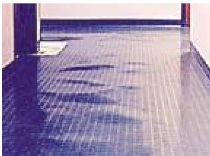
Fig. 1: Many flooring failures result when high moisture levels and a high pH beneath low-permeability floor coverings combine to produce adhesive failure
