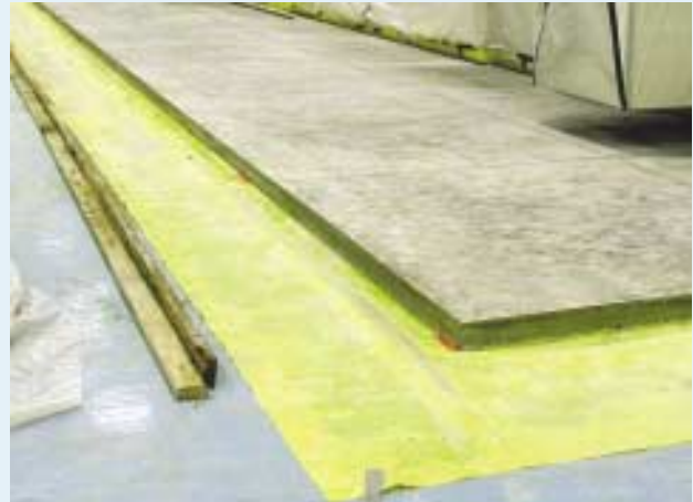
If an existing slab was built with no vapor retarder beneath it, a new slab, placed over a vapor retarder, is one renovation option
