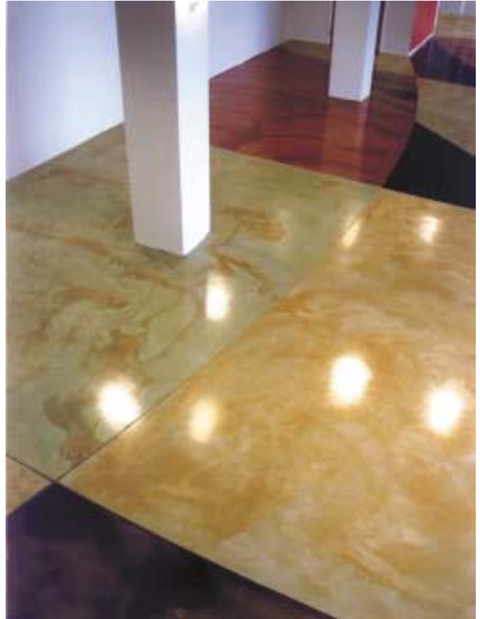
Fig. 7: Stained cementitious overlays provide a durable, decorative surface for concrete slabs on and above grade. They allow the designer and owner almost unlimited options as to patterns and colors (photo courtesy of Ardex, Inc.)
