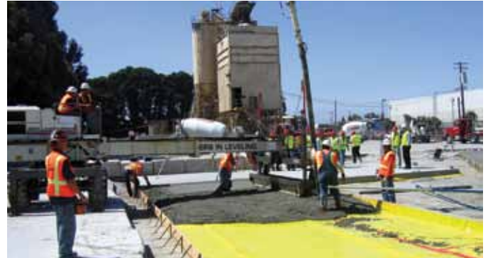
Fig. 6: Testing moved from the laboratory to the field to verify that the new concrete mixture could be placed and finished using modern equipment. Here, the mixture is being delivered using a concrete pump and being struck-off using a laser screed
